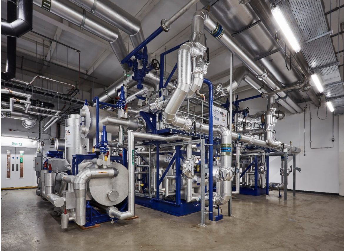
Figure 3: Photo of Ammonia heat pump harvesting heat from the Clyde estuary
